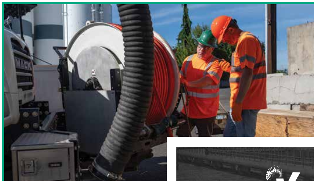
Yakima Utilities wastewater maintenance specialist Rich (left) and water maintenance specialist Shane Jones flush a sewer line.
