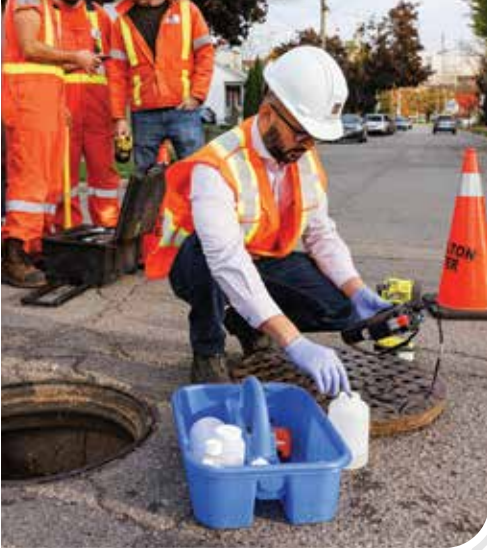
Monitoring & Enforcement Operations Supervisor Muhammad Mujtaba analyzes a water sample taken from a manhole chamber after a video inspection revealed an uncharted connection.
