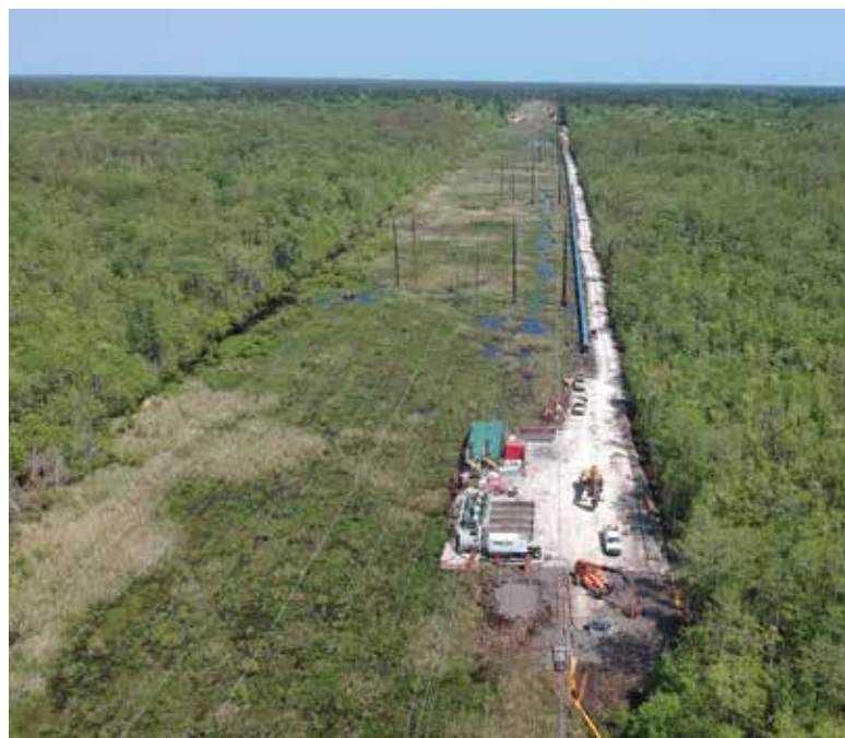
The Grand Strand Water & Sewer Authority's recently installed 48-inch-diameter water transmission main transports water from Bull Creek Surface Water Treatment Plant to the city of Conway and two other unincorporated communities.
