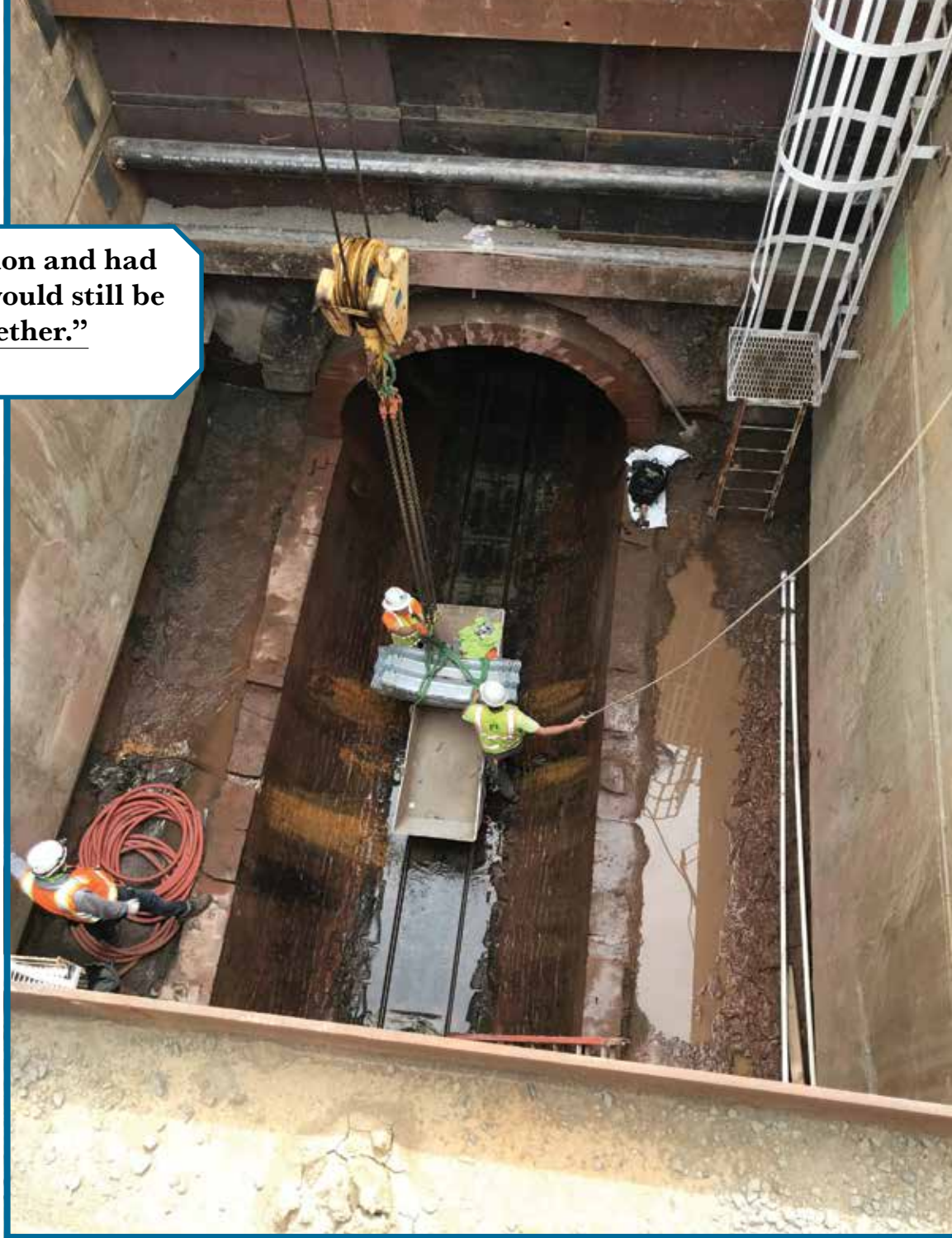
The 6-mile-long Taggart Outfall, built of brick 115 years ago, was sliplined with short sections of fiberglass-reinforced pipe.
