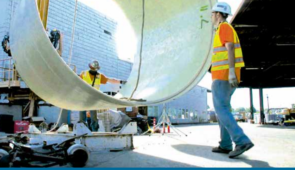
A 108-inch-diameter section of fiberglass-reinforced pipe is maneuvered into place during sliplining of the Taggart Outfall in Portland, Oregon.
